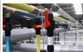
Special colored pipes
